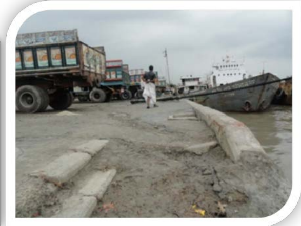
Figure 2: Figure shows the tide protection embankment at Railway Kastom Ghat area. Earlier it was about 1-2 ft. high from the high tide level but now it becomes flooded due to tidal influence. The sediment signature shows the flooding condition of the embankment BIWTA Kastom Ghat .
