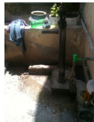
Figure 10 Hand-pump in peri-urban residence
