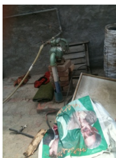
Figure 9 Electrical water motor pump
