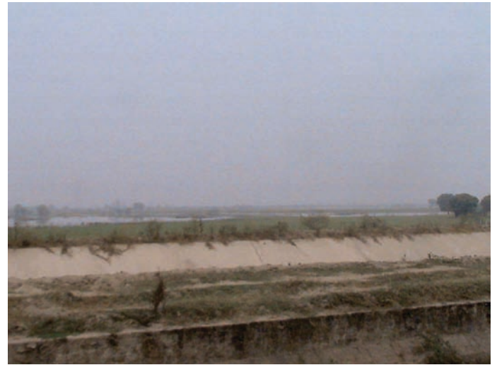
Fig.7 The NCR channel being dug to augment Gurgaon's water supply cuts through Budheda village - the villagers lost their lands to its construction)
